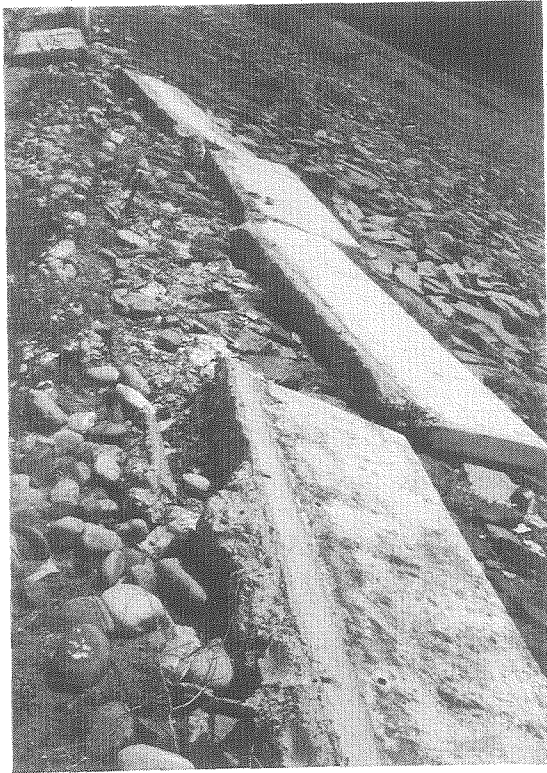
Photo 2; Overturning of concrete panels at the top of the downstream slope, La Villita Dam.
