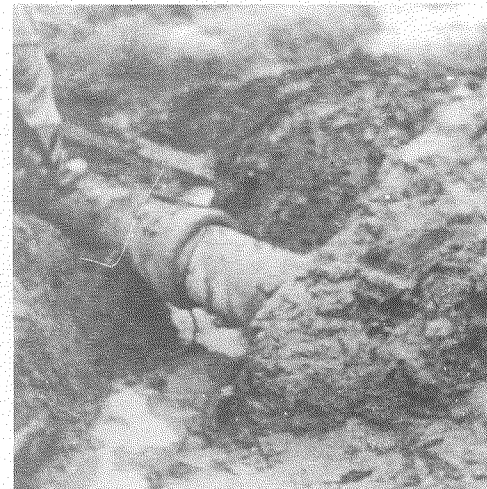
19. Pipe Damage Possibly Caused by Imposed Axial Strain (2)
