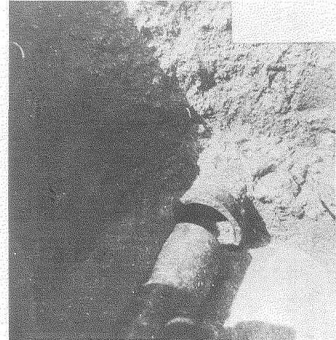
5. \phi 300 Castiron Pipe Damaged in Tangshan (2)
