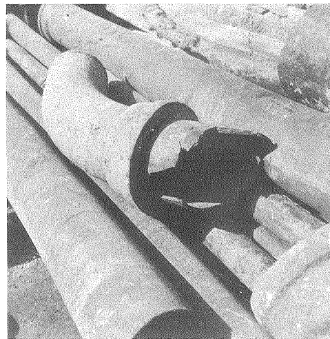
23. Damage to Pipe Fittings (1)
