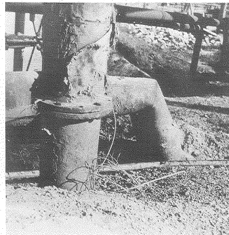
11. \phi 500 Steel Pipe in Hangu Showing Similar Damage as in Photo 10
