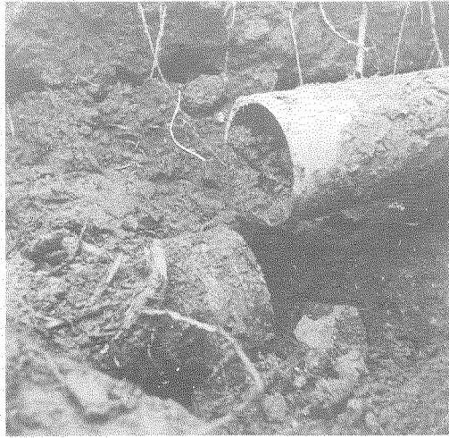
2. \phi 200 Pulled-out Castiron Pipe Showing Stagger in Tangshan
