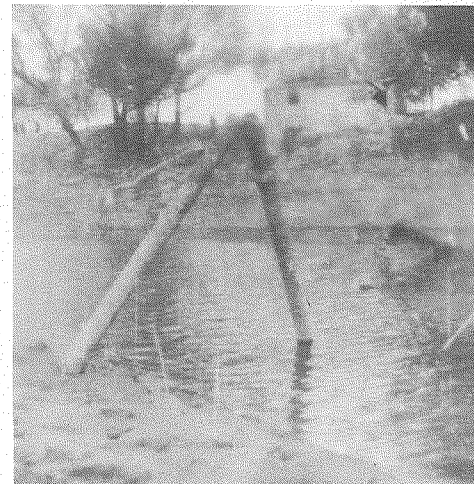
13. Buckled Steel Pipe due to Shortening Caused by Inward Bank Slides in Tangshan
