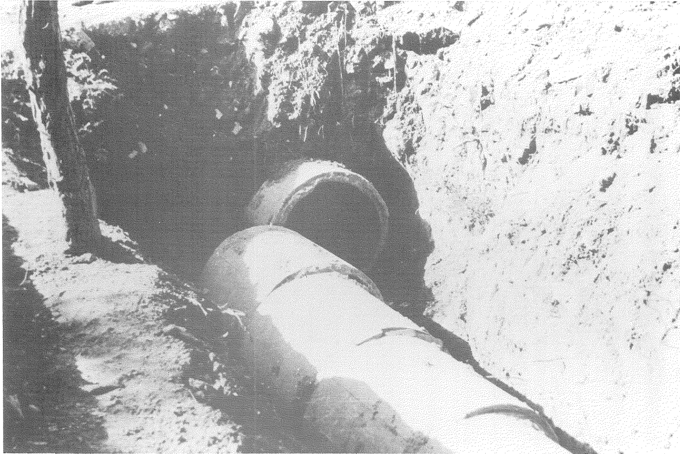
1. \phi 1000 R/C Pipe Undergoing Horizontal Stagger in Fault Rupture Zone in Tangshan
