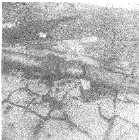
18. Pipe Damage Possibly Caused by Imposed Axial Strain (1)
