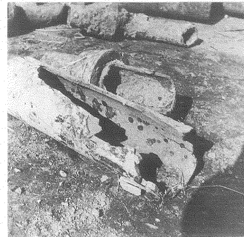
27. Damage to Corroded Castiron Pipes in Yingkou (2)
