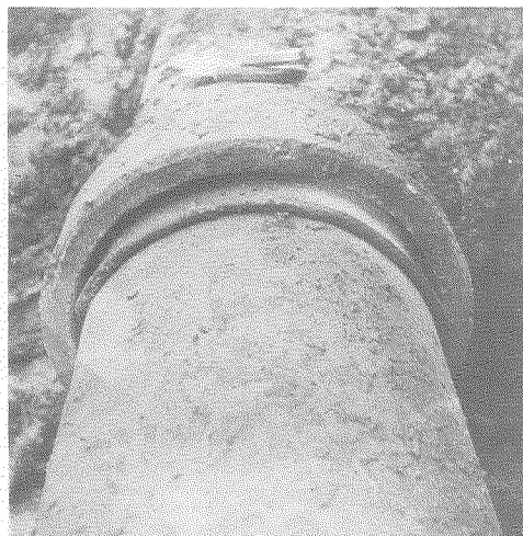
20. Pipe Damage Possibly Caused by Imposed Axial Strain (3)
