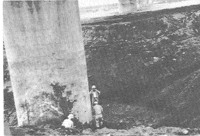
Photo. 6 A Trench Dug Around A Pier of Yuriage Bridge
