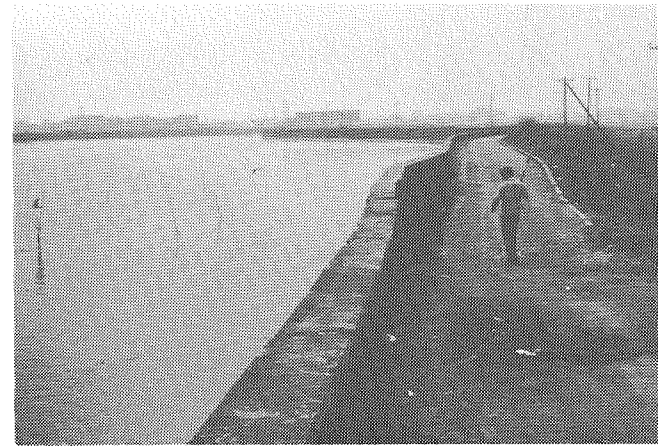
Photo. 4 Tilted Retaining Walls and Settle Road Faces Along Torino Umi
